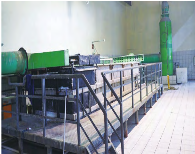
Acid-base mist treatment tower
