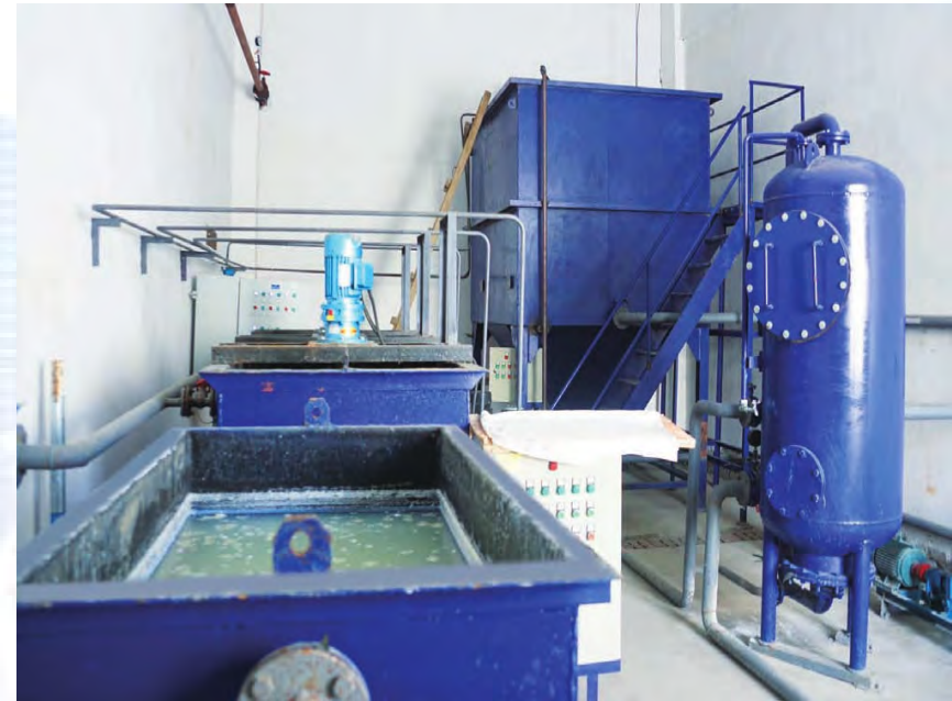
Acid and alkali wastewater treatment station
