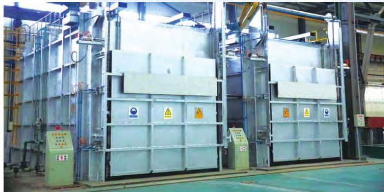
Soaking furnace group
